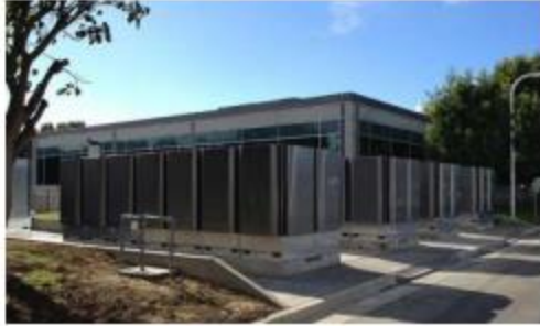
Bloomenergy – 200 kW SOFC – California, USA
